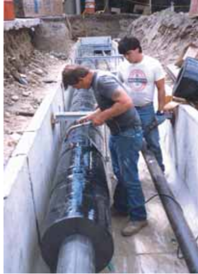
Installing Pittwrap® jacketing over Foamglas® insulation in a buried steam transmission application.
