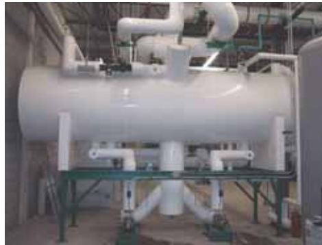
Styrofoam® brand foam insulation used to insulate a vessel.
