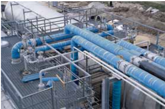
Trymer® brand foam insulation used to insulate piping in a freeze protection application.
